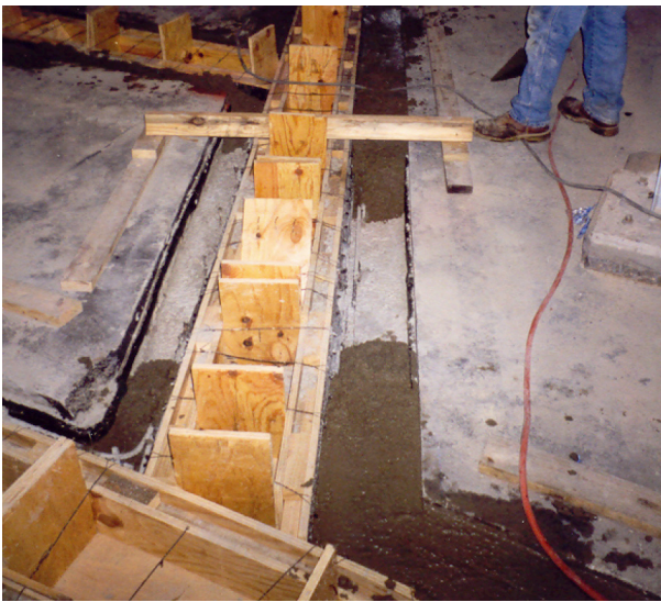
10. Sand bags are removed before the second lift of concrete is installed. The sand bags are no longer necessary, because the first lift of concrete has locked the liner in place, so it won't float.
