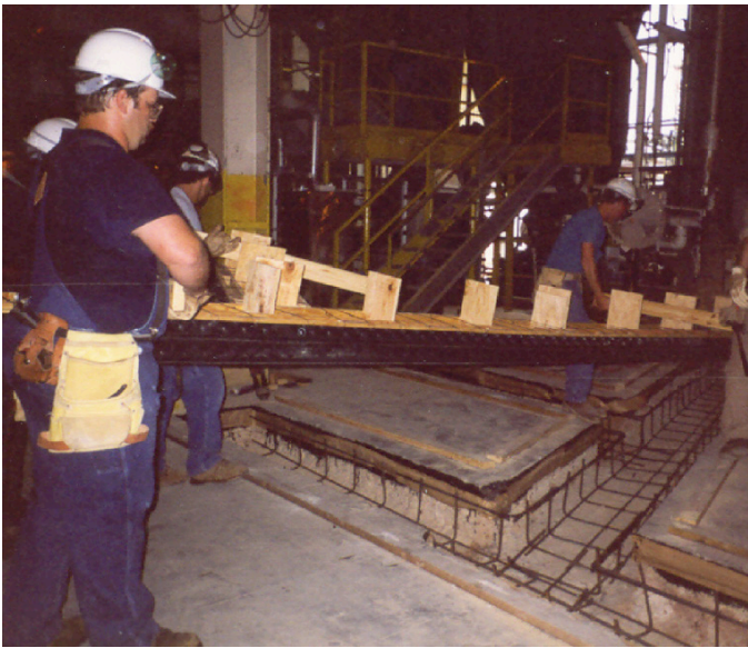
5. Workers carry the trench liners into the construction area by the 2 x 4 cross beams.
