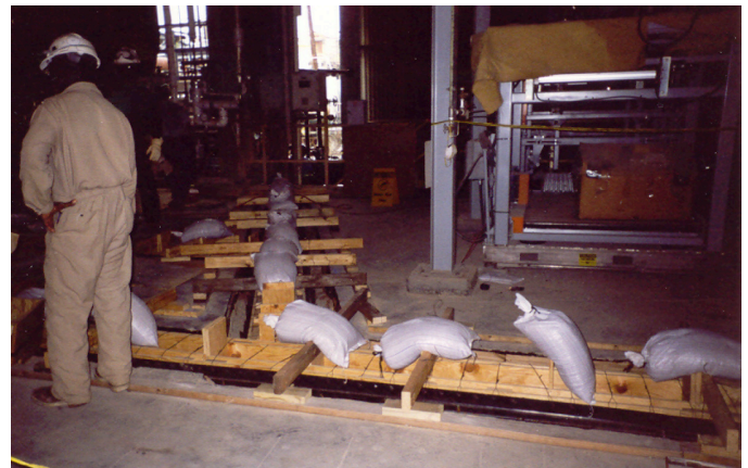
8. Sand bags are set on the trench liner formwork to help prevent the liner from floating during casting. The liner is cast in two lifts, with the first lift coming just to the bottom of the trench liner to lock it in.
