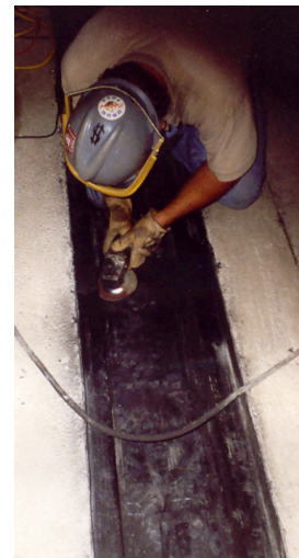
12. A worker grinds a seam area in the trench. Polyethylene must be clean, dry and scraped prior to welding. The scraping or grinding removes the layer of oxidation that forms on the surface of the plastic and could adversely impact weld quality.
