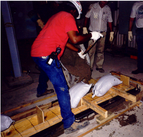
9. Workers shovel the first lift of Portland cement concrete (pea gravel mix) into the space between the trench and existing concrete.
